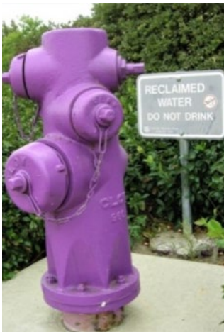
Purple pipes indicate recycled water infrastructure
