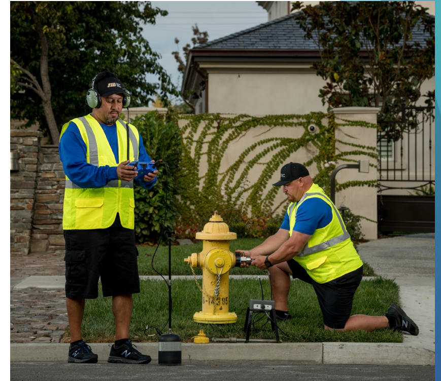
Leak Detection at SJW
